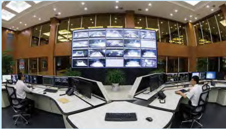
Shangwan Coal Mine's centralized supervision and monitoring platform in Shendong Coal Group
