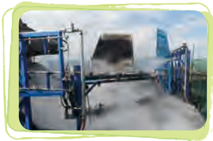
Windproof dust suppression net and dry mist dust suppression device at the crushing station
